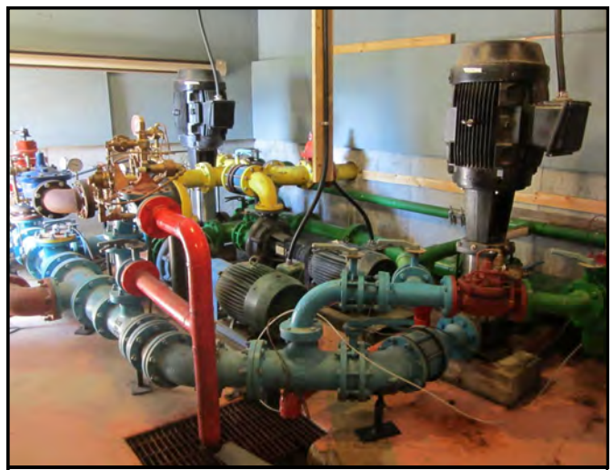
1750 & 1990 reservoir booster pumps
