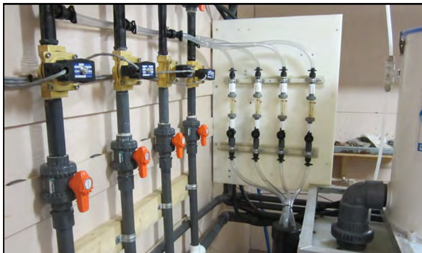
Main Chlorine application system
