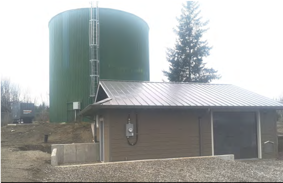
1990 Highlands Phase 3 Pumphouse & Reservoir with Emergency Power Generator
