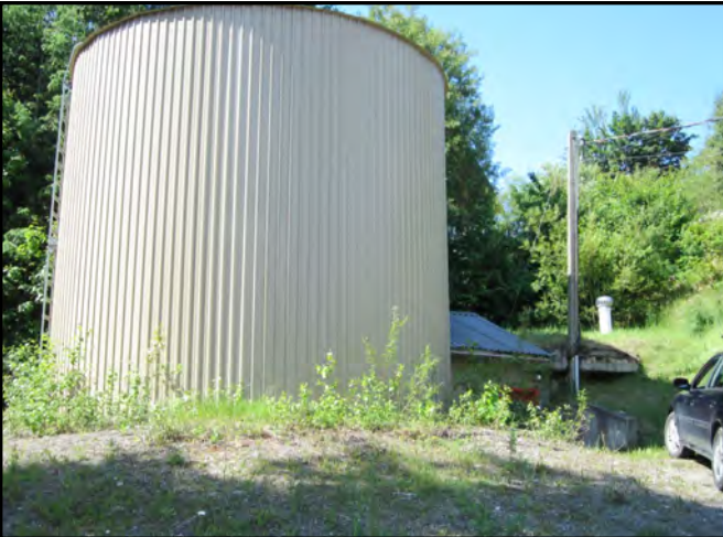
Waverly Drive reservoir & booster pump house
