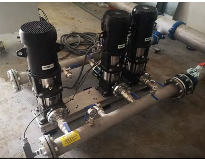
1990 Domestic water pumps
