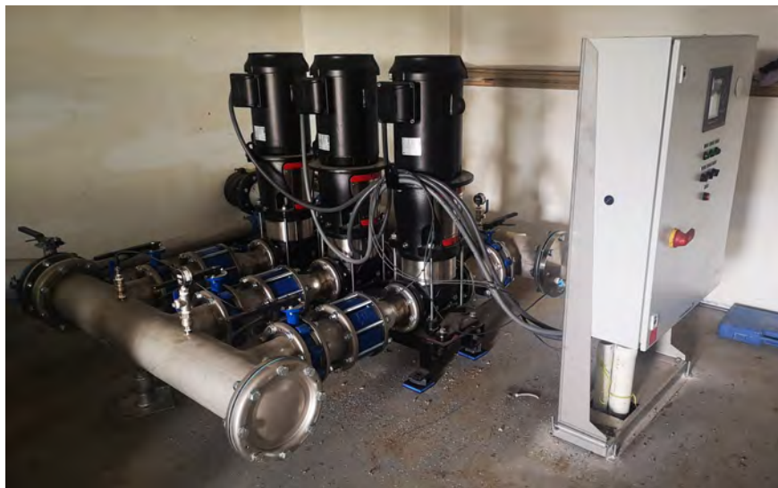
1990 Fire water pumps
